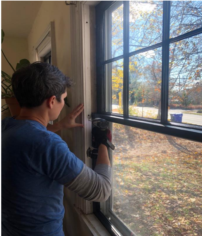
Fitting a newly restored lower sash; the top sash has been fixed permanently inoperable, and sealed tight.
